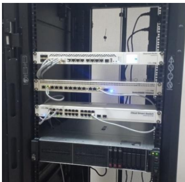
Figure 4. MikroTik Backbone Used (Router Number 2 RB 1100 AHx)
