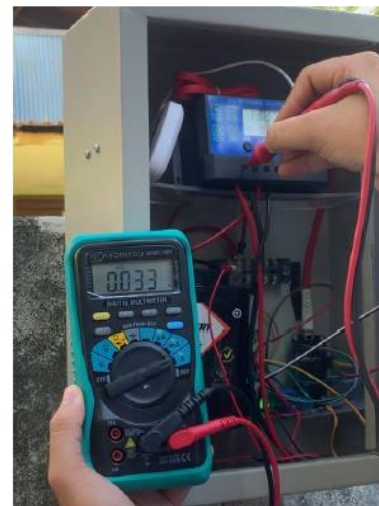
Figure 12. Solar Panel Testing
