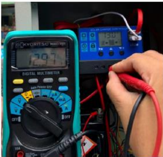
Figure 14. Battery Battery Testing
