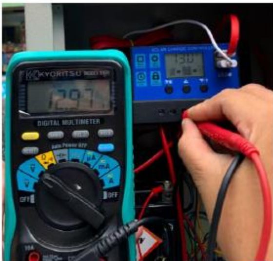
Figure 14. Battery Battery Testing
