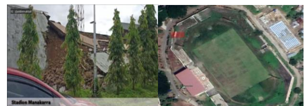
Figure 13. Damage Detected at Manakarra Stadium
